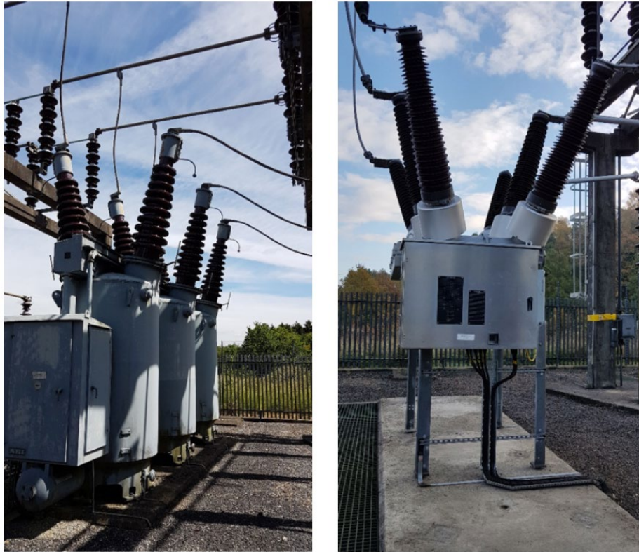
Figure 1 – Example replaced 132kV CB - AIB (OD) at Amersham Main Old Oil (Left) New SF6 (Right) 1
