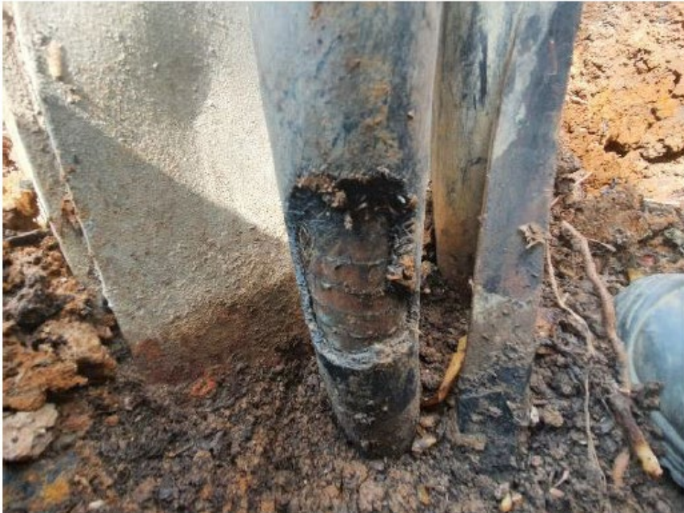
Figure 2: Rodent damage to outer sheath of 132kV FFC in Fleet, on the SEPD network
