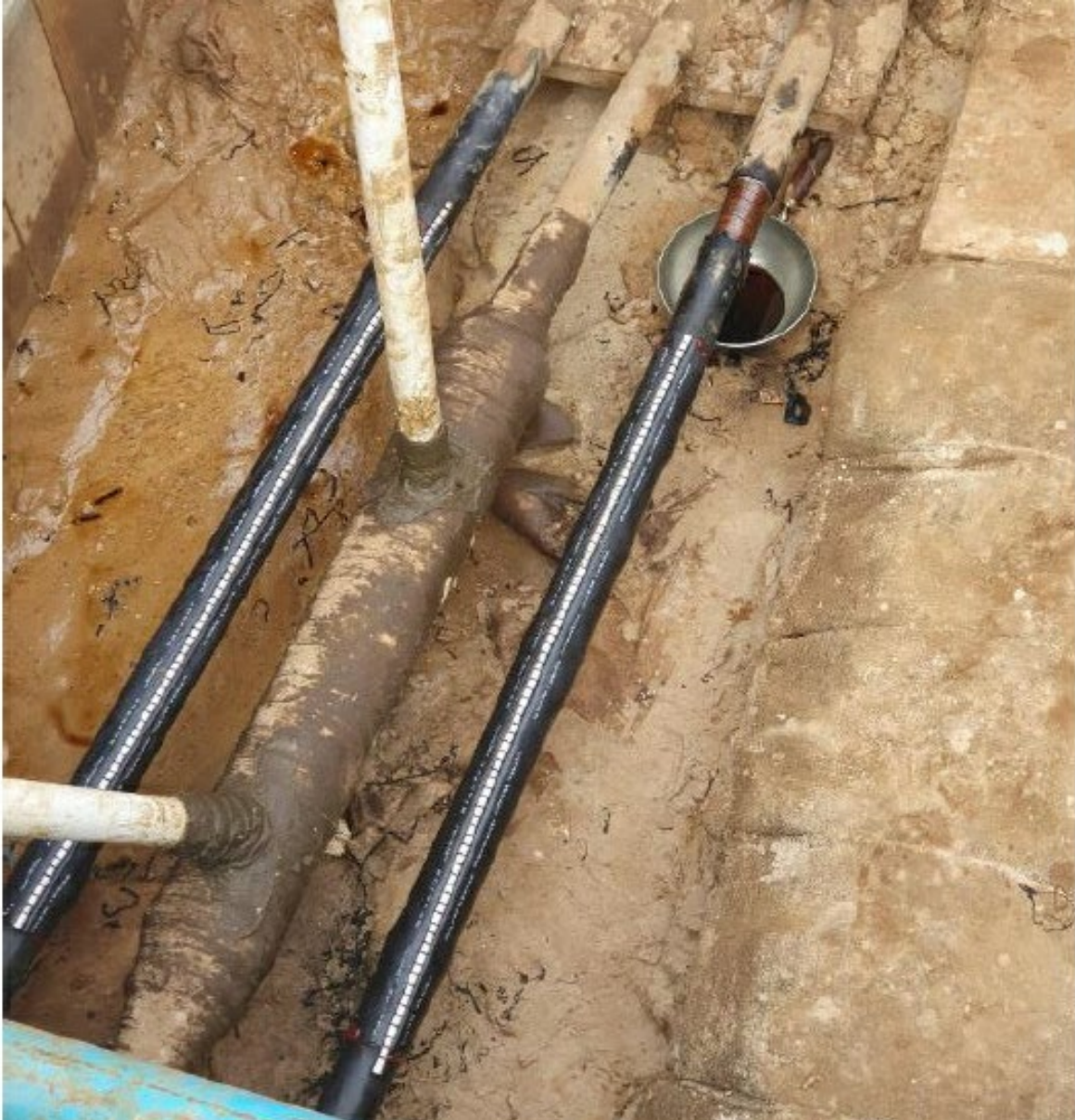
Figure 1: Leak identified on 132kV FFC in Fleet, on the SEPD network
