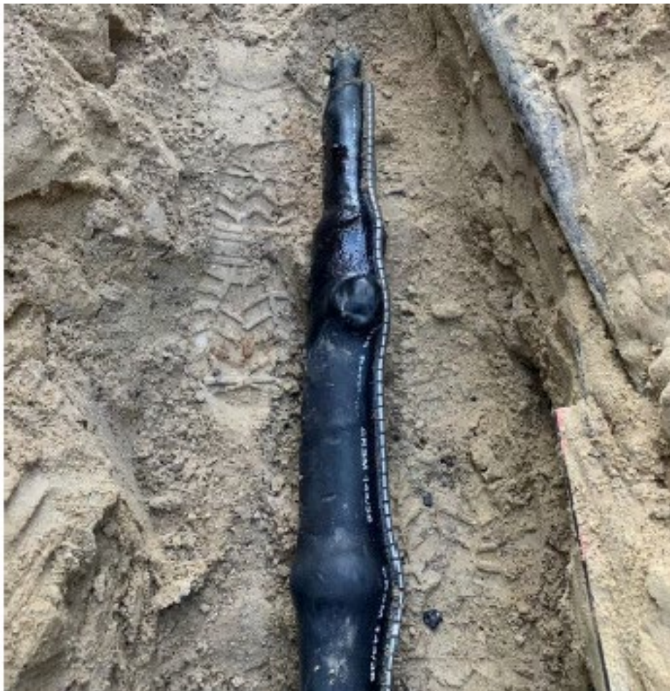
Figure 3: Previous repair can to FFC in Christchurch showing signs of leakage
