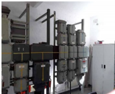
Flashguards inside Electrical Boxing
