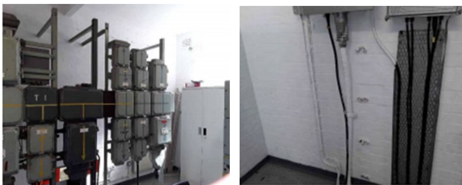
Figure 1: Examples of ACM (Flashguards inside Electrical Boxing and Cable Wrap)
