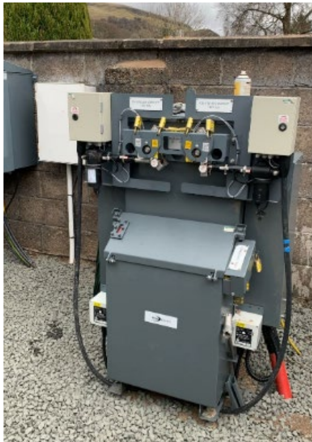
Figure 2: Automated RMU with Actuators & FPIs
